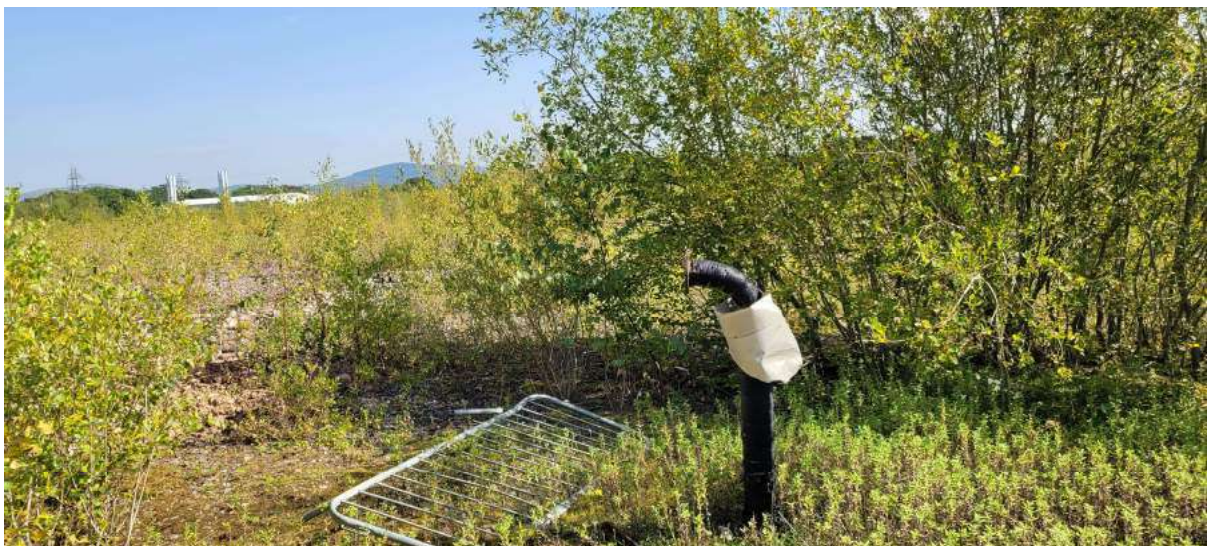
Suspect Steam Pipe Network
