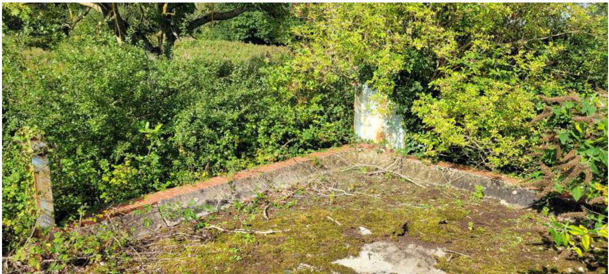
Former Building Position – Undocumented Retaining Wall
