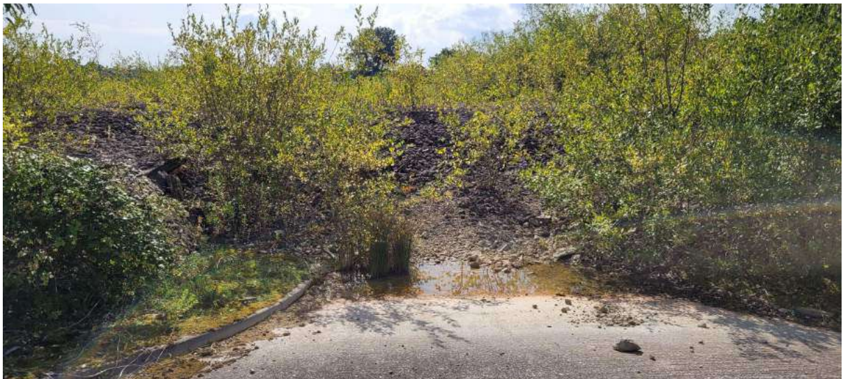
Ramp/Change in Level from Demolition Debris
