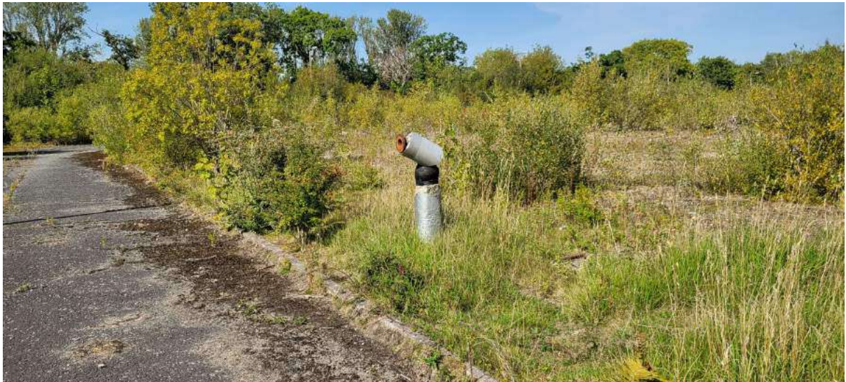
Suspected steam pipe network
